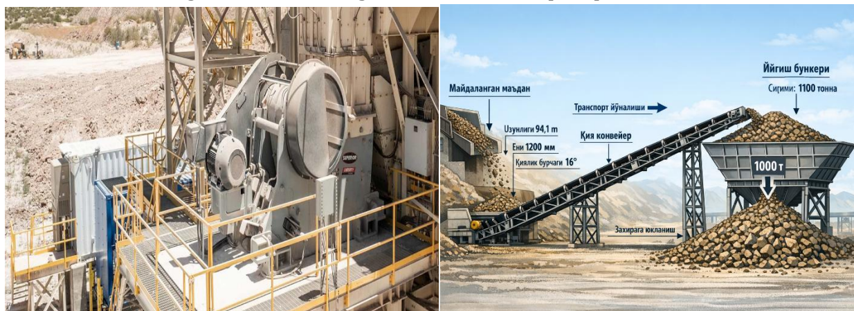
Figure 3. SHDP-12×15 type crusher and conveyor
